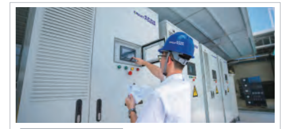
Guangzhou Xinli 2.33MMh Project
