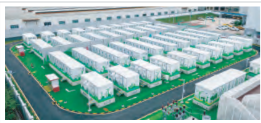
Nanning 100MMh Energy Storage Project
