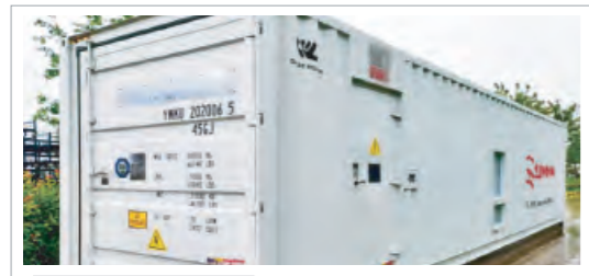
Croatia 17MMh Photovoltaic and Storage Complementary Project
